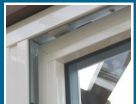
Secure Night Vent Facility
